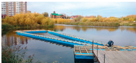
2015. The winter bathing and cold water treatment club «Kristal» in Tyumen is constructing a hypaethral swimming pool from the floats produced by our company. To make the pool, the club bought 52 floats - for the pool with the 8 m width and the 25 m length.
